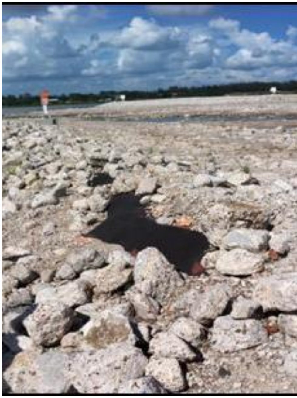
The armored cap at SJRWPs (Texans Together)
